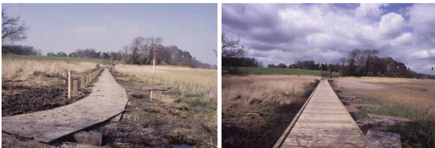
Fig. 8 – Boardwalk under construction and on completion c 1987/8 showing degree of trampling and ground disturbance
